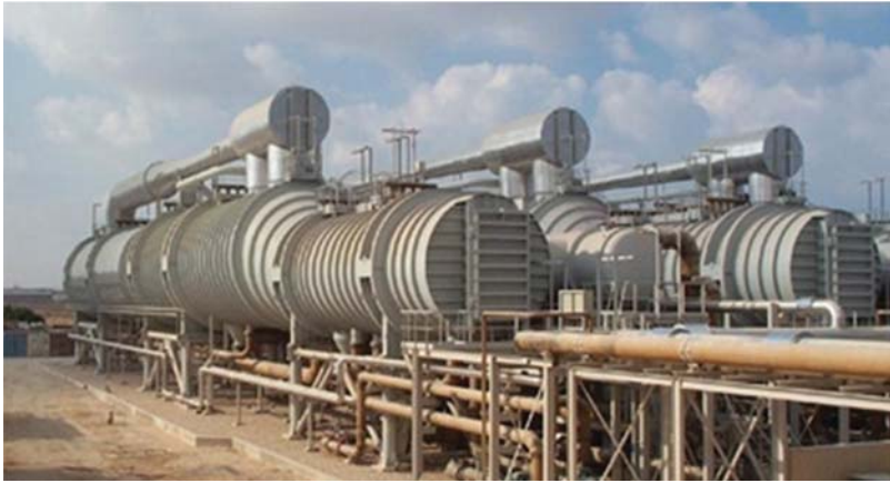
Figure 2.56 MED - TVC plant with 3 units each 13,333 \text{ m}^3/\text{d} / Tobruk, Libya (by courtesy of SIDEM (VEOLIA Water Systems) [14].
